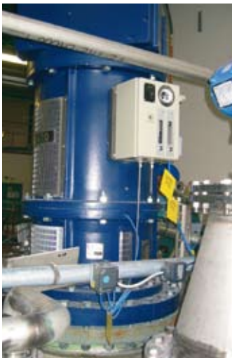
Glass-lined polymerisation reactor (Ekato) for producing ion exchanger granules at Lanxess Bitterfeld, Energizing Chemistry.
