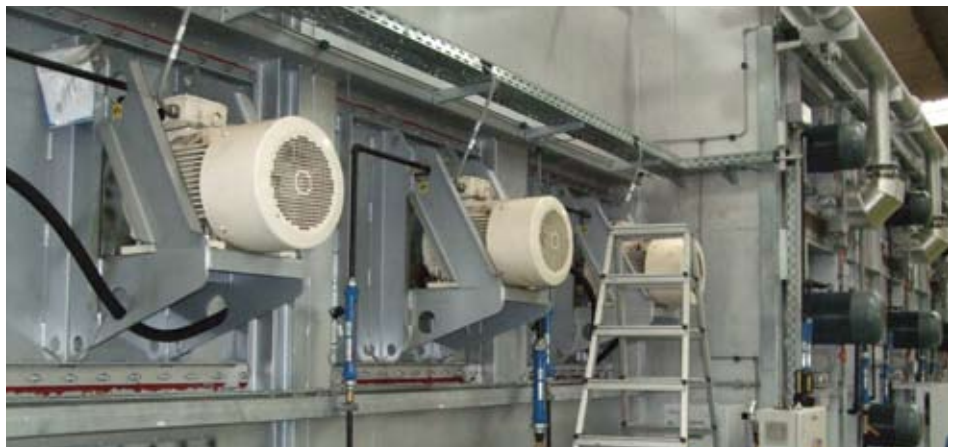
Continuous kilns' fan drives for the heat treatment of metal strips Photo by courtesy of Aurubis AG
