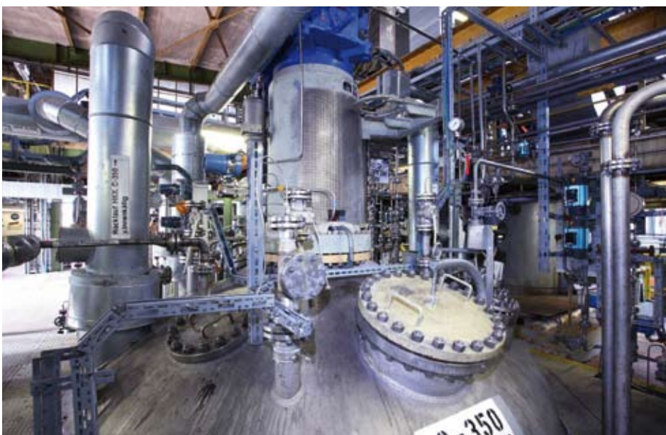
Agitator in a chemical plant
