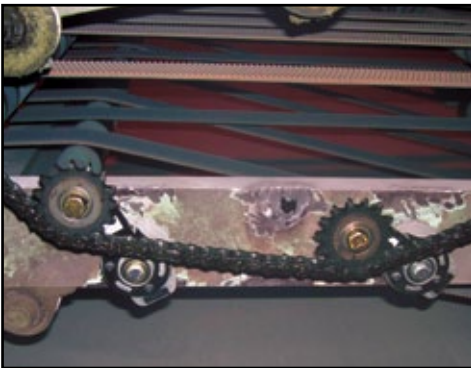
T-Max® Tensioners mounted on a drying oven
